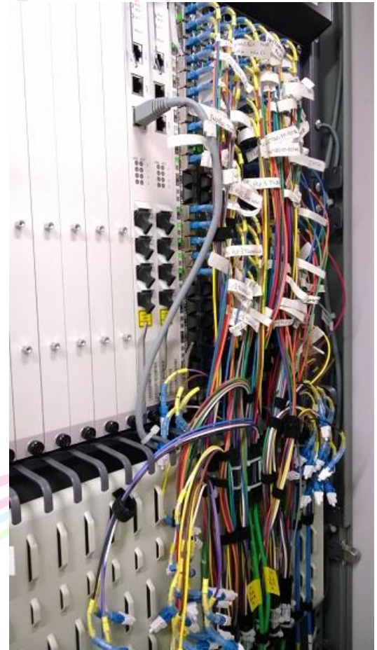
Optical Line Termination
