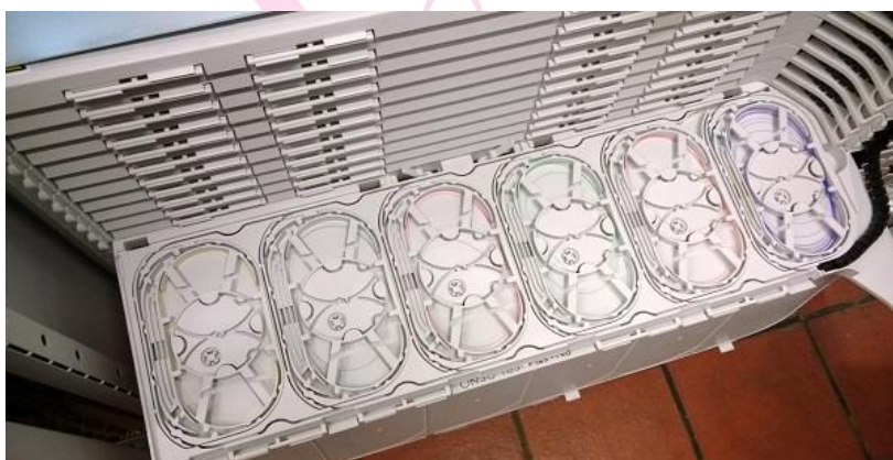
Optical Consolidation Rack: The trays wrap the individual fibres.
